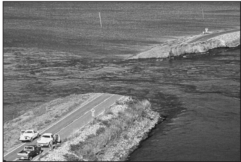
Sudden dry weather failure of Middle River Levee on Upper Jones Tract near Stockton in 2004.
